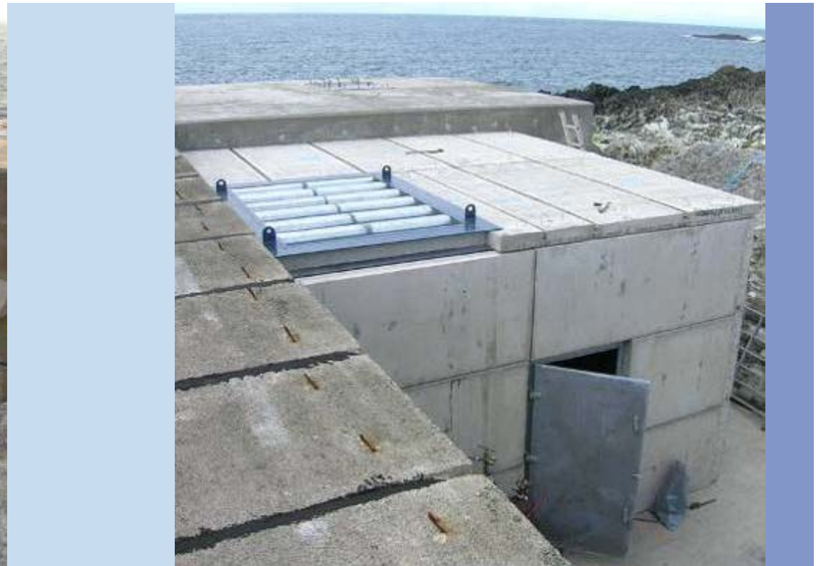
Turbine hall & acoustic attenuator
