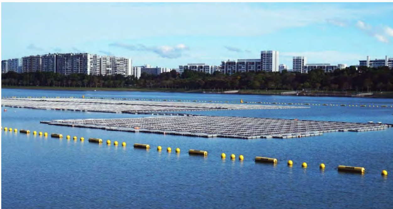
Floating Solar System in Reservoir
