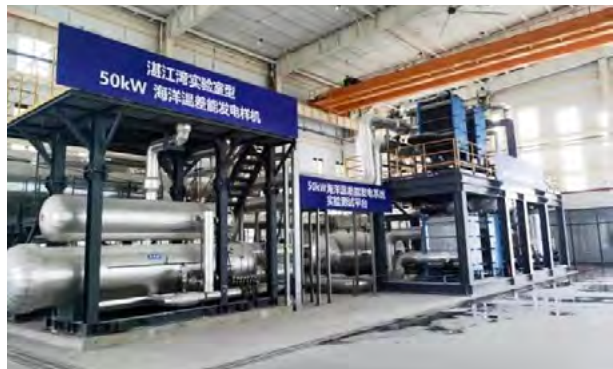
50 kW OTEC generation system and experimental test platform
