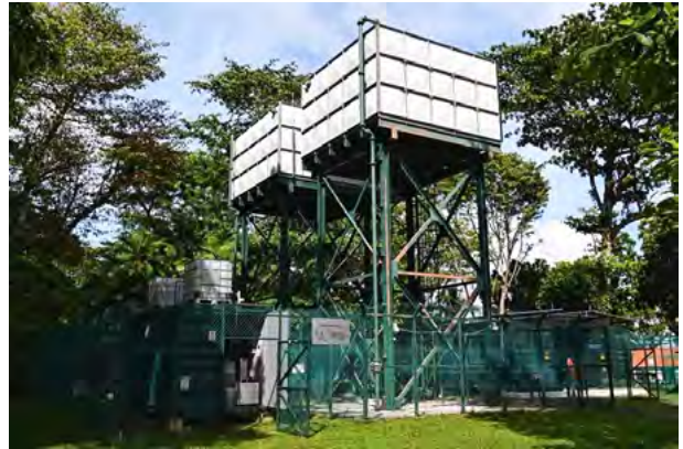
Renewable powered water generation system deployed in Kusu Island, Singapore
